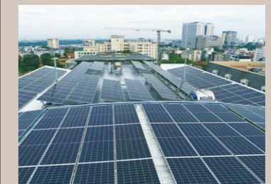
Solar panels installed on the rooftop of the CornerStone Building
